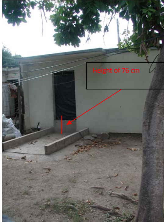
Plate 10: House near the drains in Caymanas Gardens D
