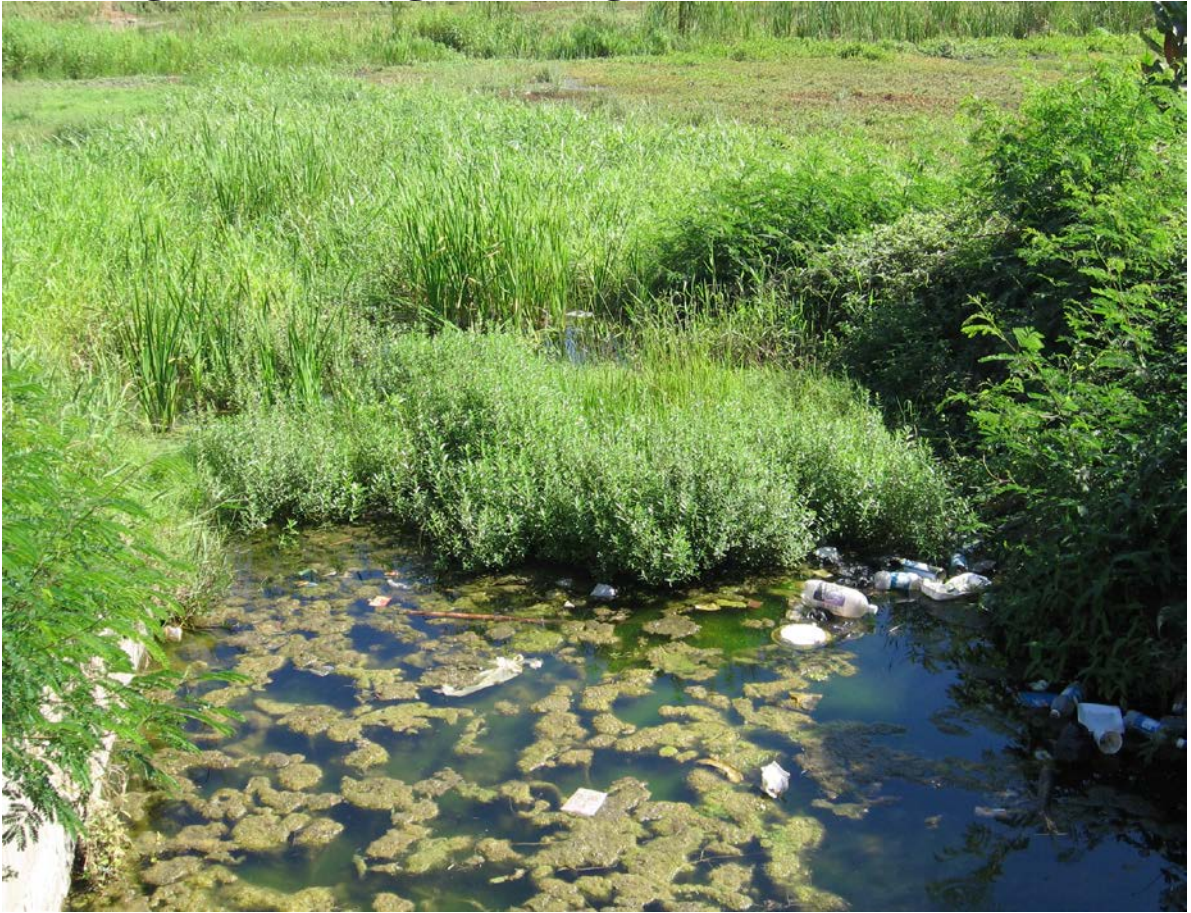
(Fig: 6) Blockage due to Vegetation Overgrowth
