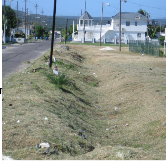
Bushing of Storm Water Relief Drain – 7 – West Greater Portmore.
