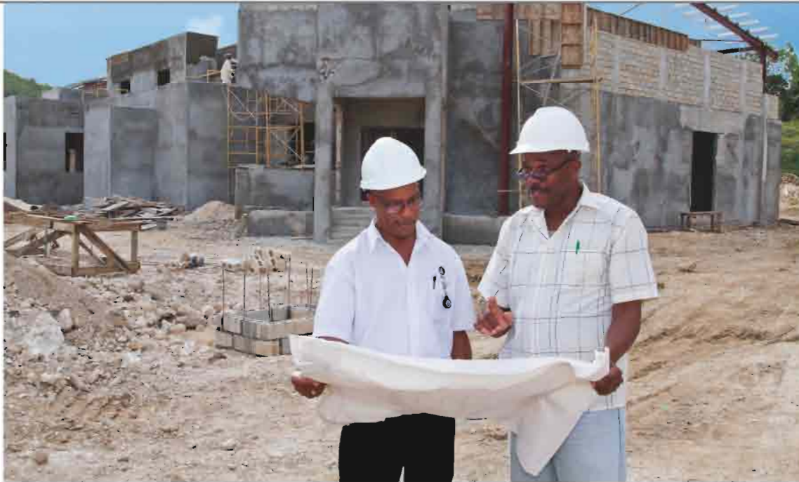
Workers at the Sweet River Abattoir that is currently under construction in Westmoreland.
