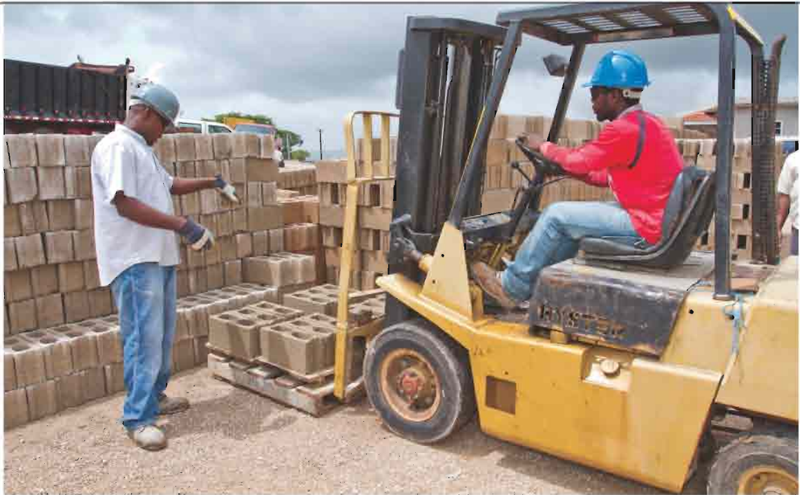
Workers load blocks manufactured at the Manchester-based May Day Block Factory Trucking Construction & Development Limited.
