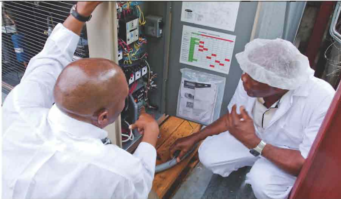
Personnel at Pioneer Meat Products Limited examine a cold storage room compressor fitted with a timer that automatically shuts down the cold storage room during peak hours as a method of energy conservation, helping the company to reduce its energy rates.
